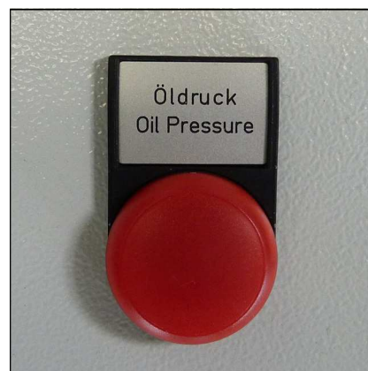
Oil Pressure Monitoring
