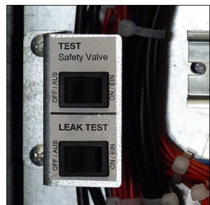
Leak test switch (lower)
