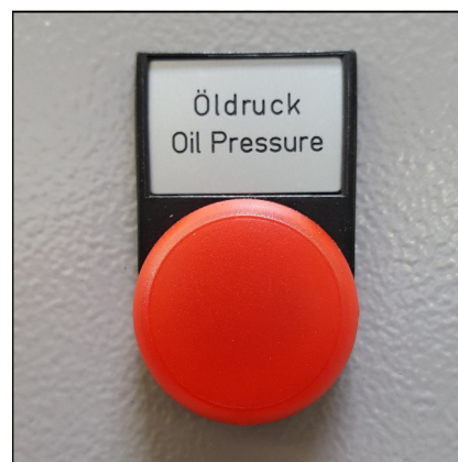
Oil Pressure Monitoring
