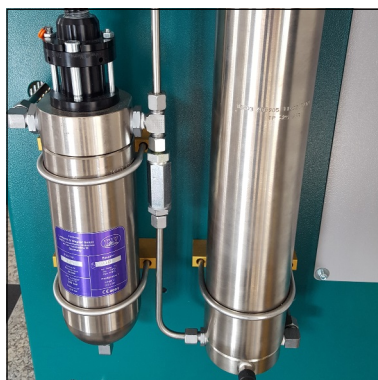
Fig. 3 - Loose pipe connections and nuts
